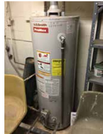
View of Hot Water Heater
