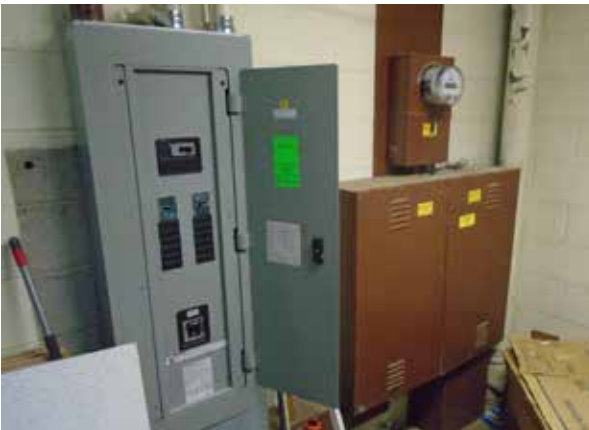
Views of Electrical Panels
