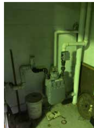
View of Gas Meter
